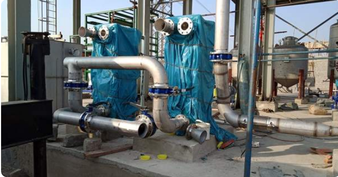
Stainless steel piping for plate heat exchangers
