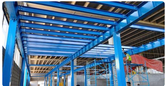
Bolted steel mezzanine framing
