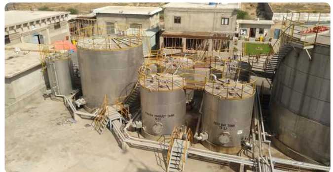
Completed tank farm with platforms and piping
